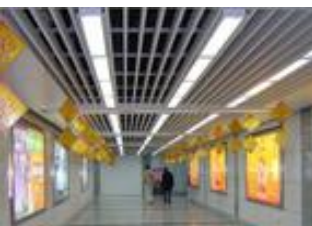
Metro Lighting Project
