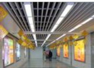
Metro Lighting Project
